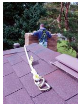
Figure 2: Roof Anchor Installed on a Roof Subsurface
